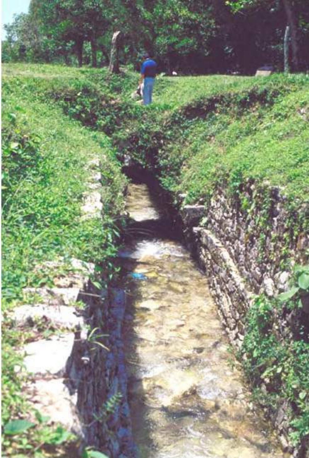
Figure 4. Ruined section of aqueduct.
