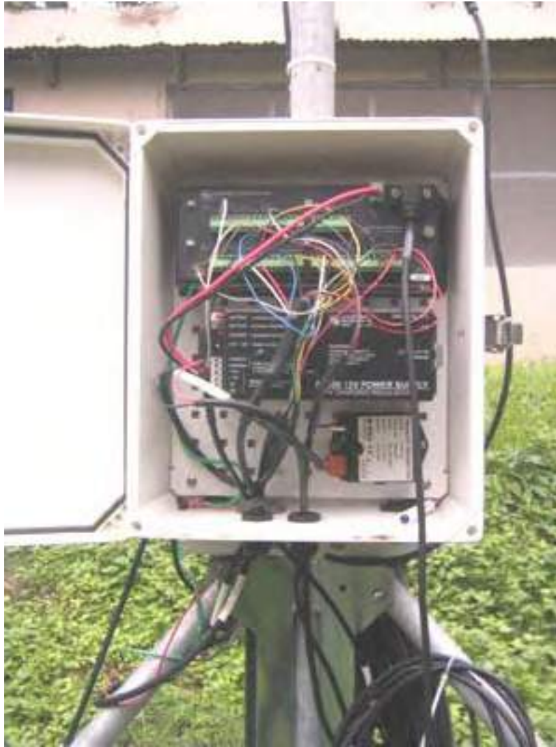
Figure 15. Interior of the CR10X Datalogger.
