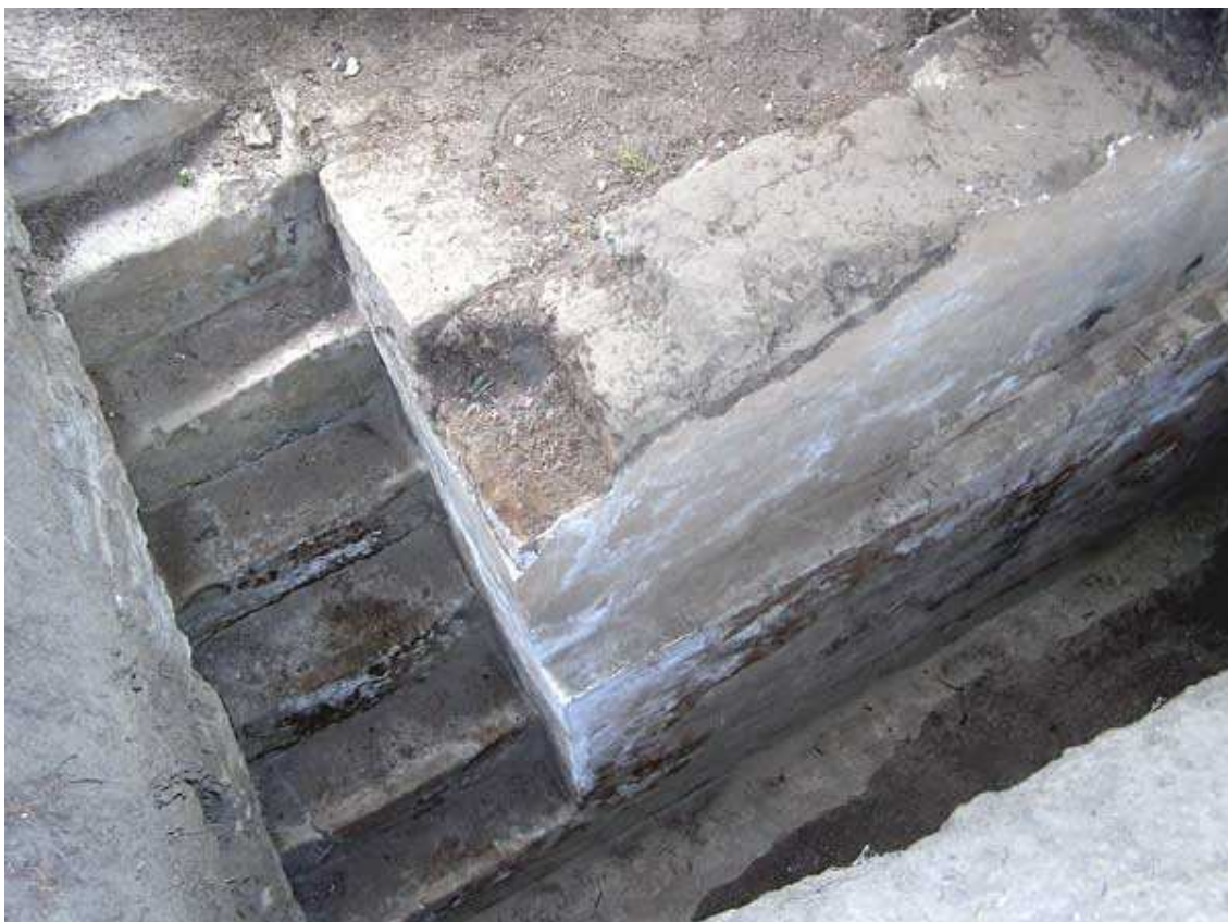
Figure 25. Wall and stairway partially uncovered in the western façade of Platform RC6a. These excavations were probably carried out in 1980.
