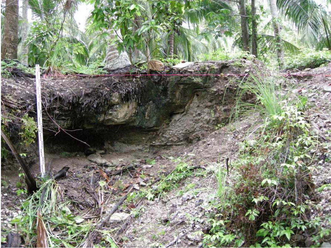
Figure 9. Feature 196 in the Northeast Group: substructure with brick and mortar vaulted arch exposed by decades old trench.
